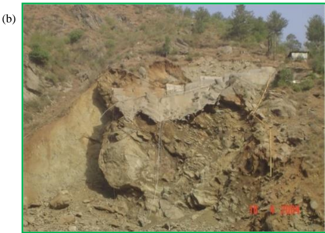
Figure 4 a,b. View of slide in the u/s of powerhouse cut slope between RD -7m and +9m starting from El±1440M to El±1368M
