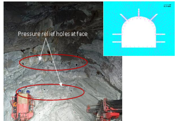
Figure 25. Drilling of stress relief holes in the tunnel of the study area to reduce rock bursting; (Inset) stress relief holes converting radial stress to tangential stress
