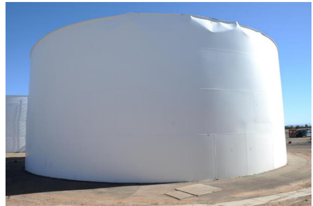
Figure 3: Damage of liquid-filled tank 2010 Calexico earthquake in California [9].
